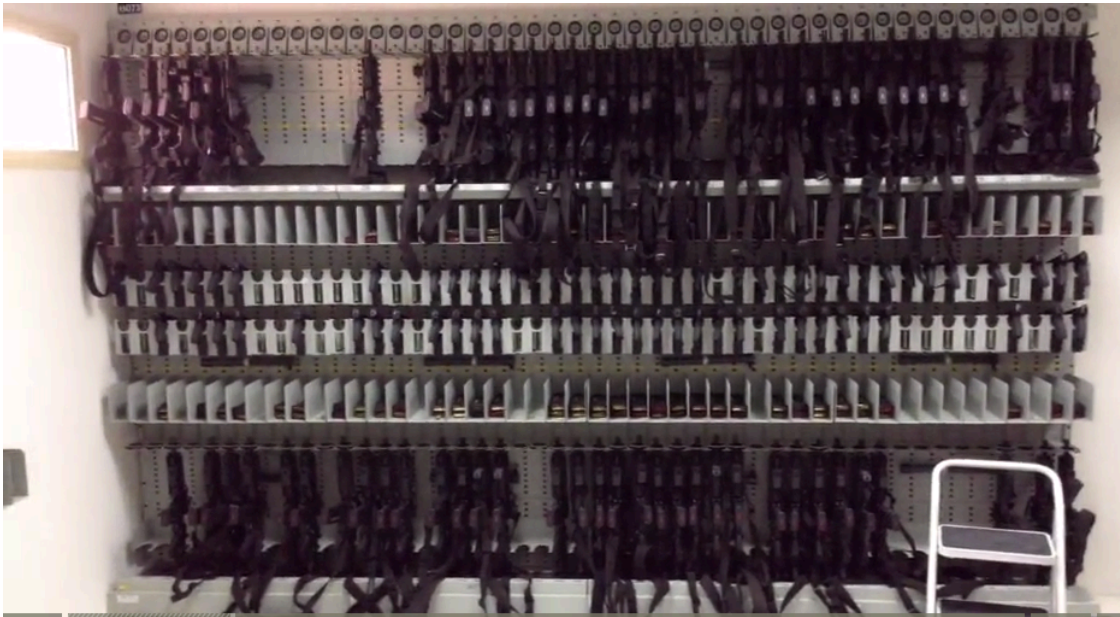
Figure 1 Site 24 - Racks 7-10 Sept. 16th
